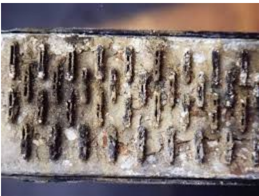
Rust, scale and sludge can plug cooling system fins, preventing proper circulation of coolant.
